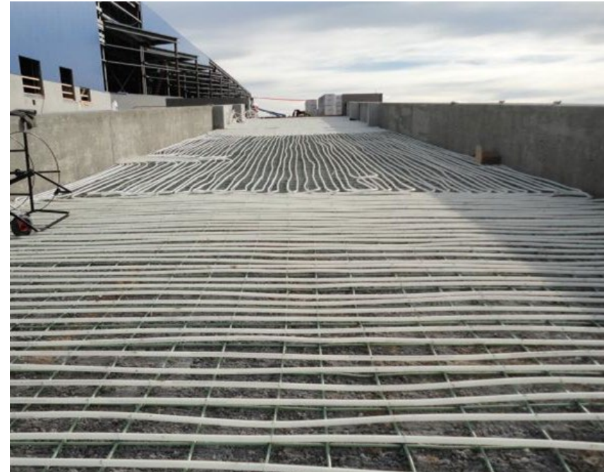
Melted Snow on Sidewalks
